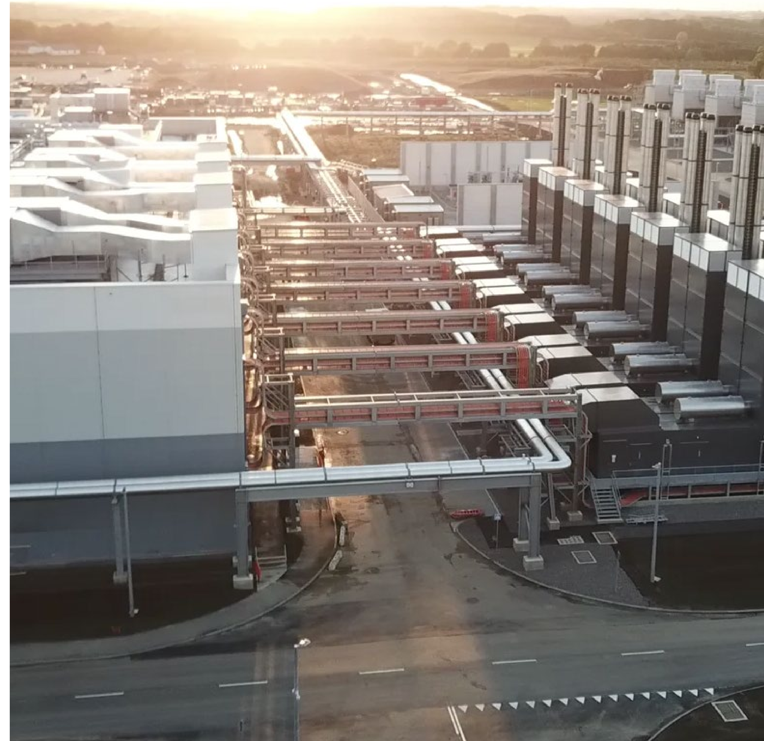
FREDERICIA DATA CENTRE, DENMARK
